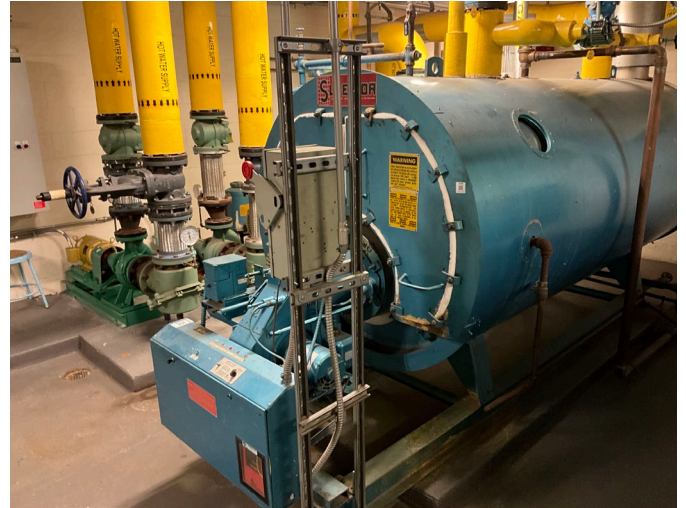
20 - BOILERS AND PUMPS
