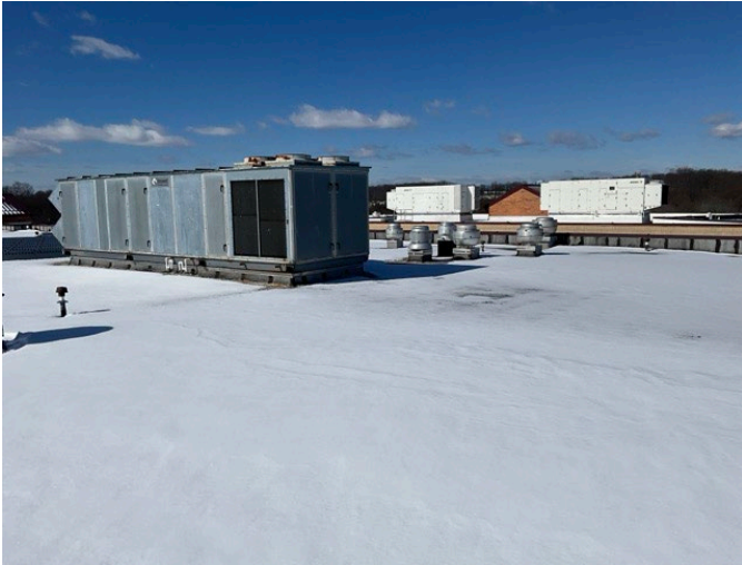
19 - ROOFTOP MECHANICAL EQUIPMENT
